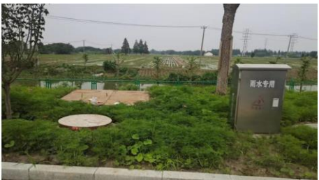
Rainfall Collection System at Luxshare Electronic Kunshan
